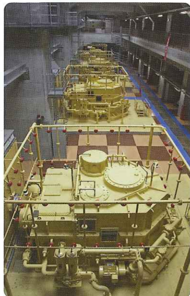
View of pump room
